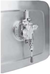
Montageposition am Tank
